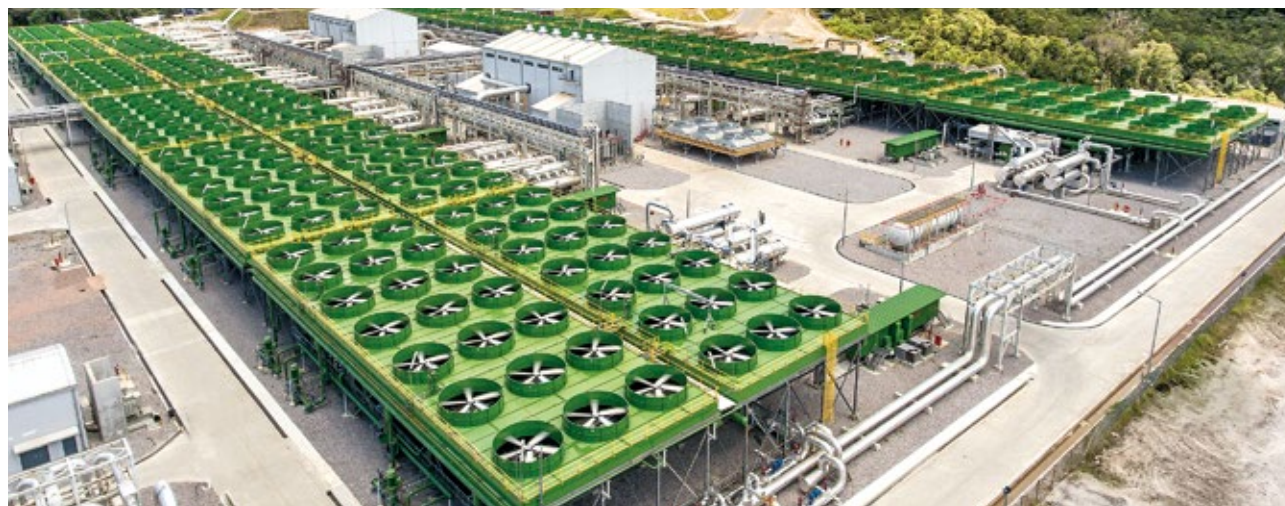
Operasi Sarulla Geothermal, Indonesia
